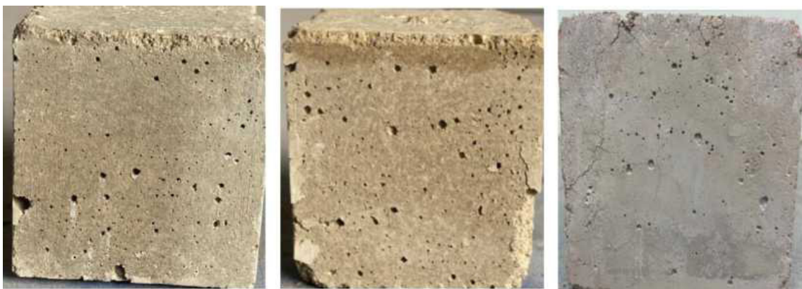
Figure 7. Surfaces of elevated temperature exposed specimens at 600 °C: (a) discoloration, (b) surface spalling, and (c) crack formation
